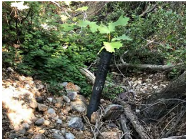
Photo 6 - Location of Spring 2 overflow and drain line outlet. The outlet is buried, and marked by the black pipe.
