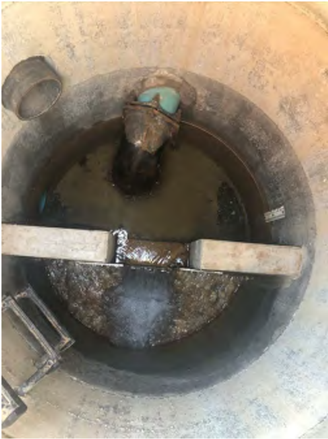
Photo 11- Spring 3 Collection box and weir
